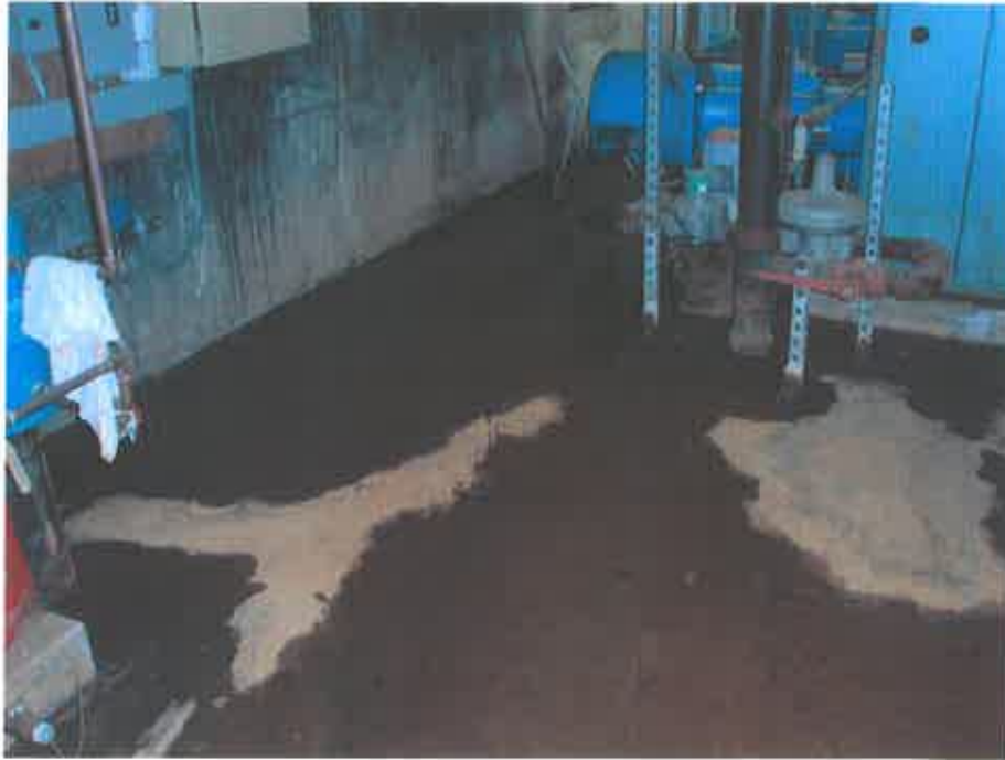
Picture 1.11. View of Smith basement boiler room, showing water infiltration.
