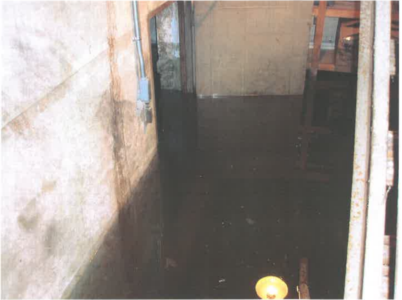
Picture 1.14. View of stairwell to the Smith basement taken on March 15, 2010. Water is 53 inches above the floor level.
